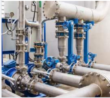
PUMP & FLUID MANAGEMENT
